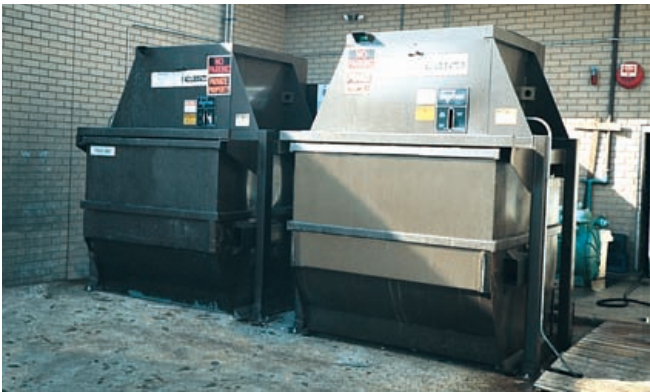
Five 8 yard VIP's, three for corrugated and two for waste, are installed at a shopping mall in Alamance County, NC. These VIP's also reduce the number of hauls through compaction, are conveniently located for mall tenants, and eliminate contamination of recyclables.
